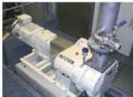
The TORNADO® T1 in use in a paper mill. Kaolin tankers are unloaded at 75 m 3 /h against a pressure of up to 4 bar.
