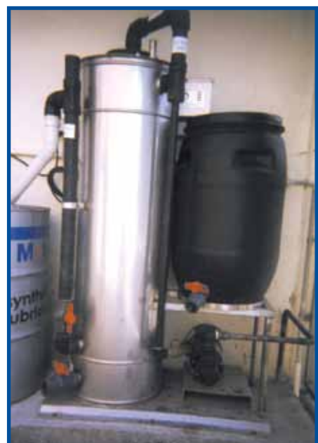
OILY WATER SEPARATOR
