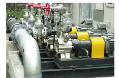
KTM Installed in parallel system
