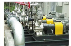
KTM Installed in parallel system
